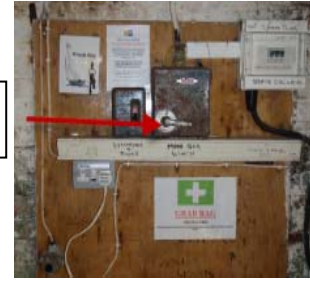
Main winch power switch
