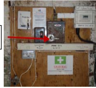
Main winch power switch
